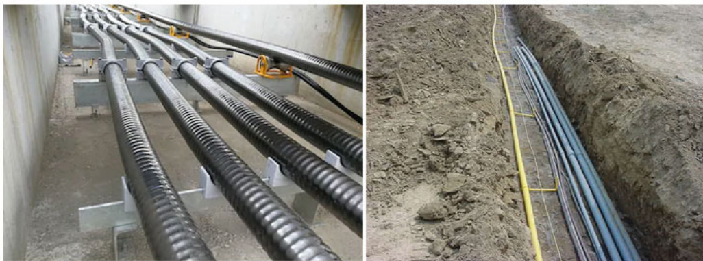
Cable Trench - With Pipe
