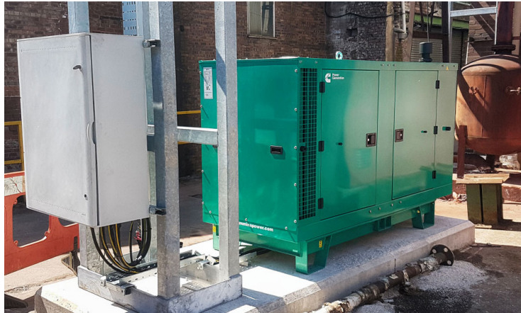
Fig. 3.1.38 Backup power sources
