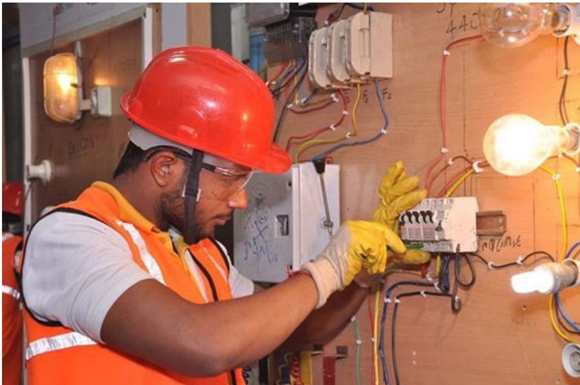
Fig. 1.2.1 Construction Electrician - LV
