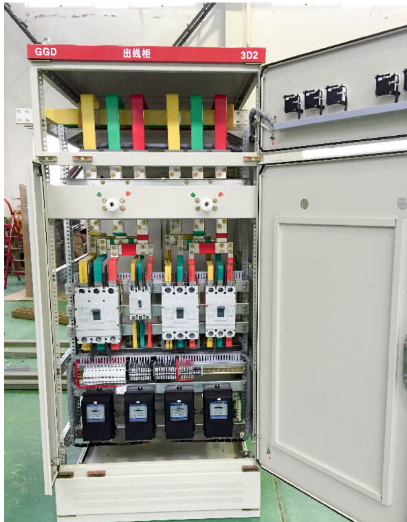
Fig. 5.1.56 Electrical distribution board (DB)
