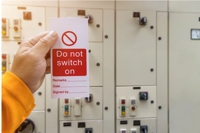
Fig. 5.3.6 Identifying issues and preventing electrical hazards
