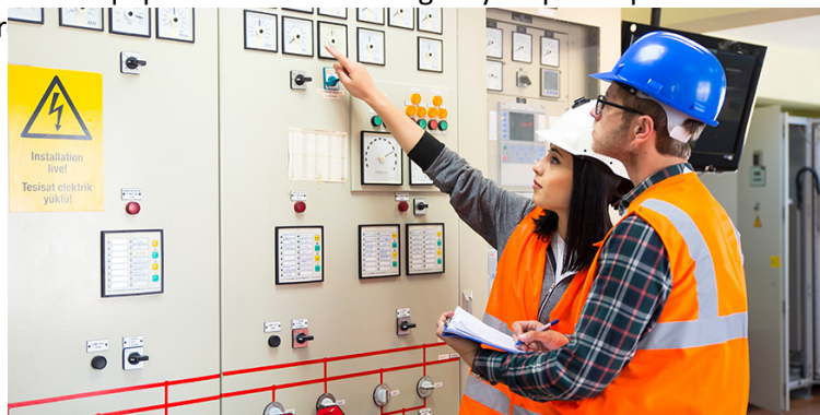
Fig. 3.1.15 Electrical safety practices
