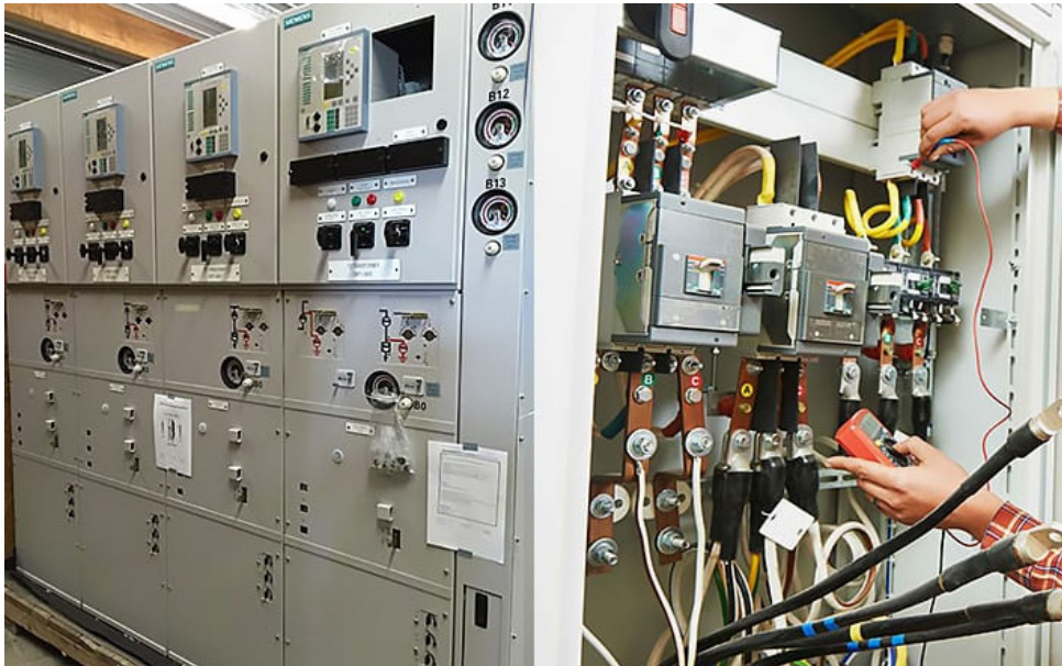
Fig. 3.3.40 Switchboards and panels
