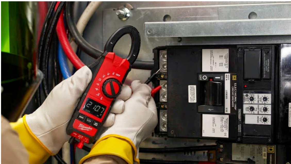
Fig. 4.2.29 Diagnosing electrical faults in construction equipment
