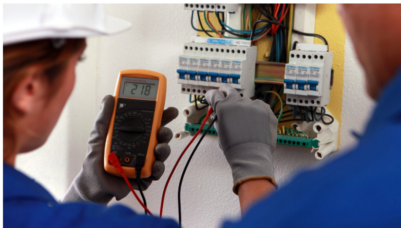
Fig. 3.3.43 Compliance of electrical installations in India
