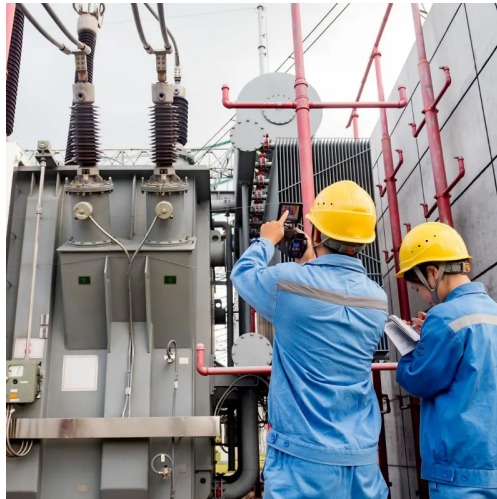
Fig. 4.2.20 Regular inspection and operation of transformers
