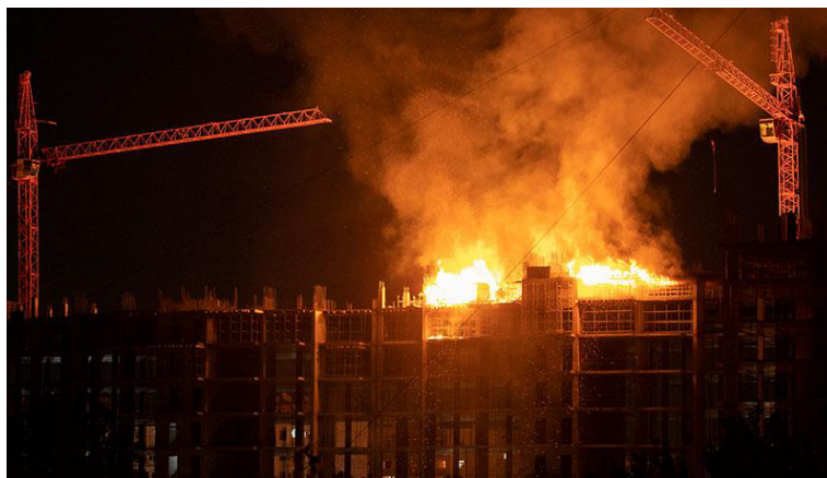
Fig. 5.2.3 Fire at Construction Site
