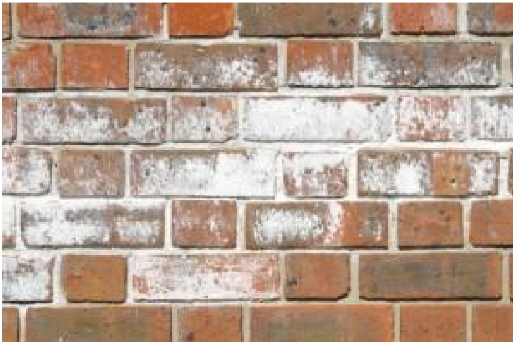
Fig. 3.1.18 Efflorescence test of bricks
